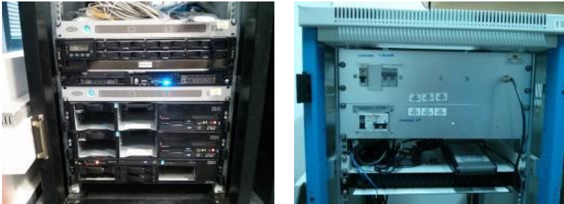
Figure 20 Detail of processing servers (left) and management/storage servers (right).
