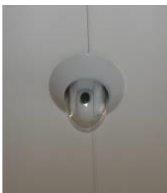
Figure 5 Detail of one of the PTZ cameras located on the ceiling of the EPS hall.
